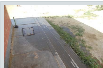
Raw Sewage Overflow at School
